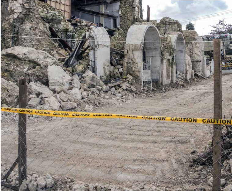
Barriers and caution tape help to warn people and secure a heavily damaged church in Philippines, 2013. Photo: Aparna Tandon, ICCROM.
