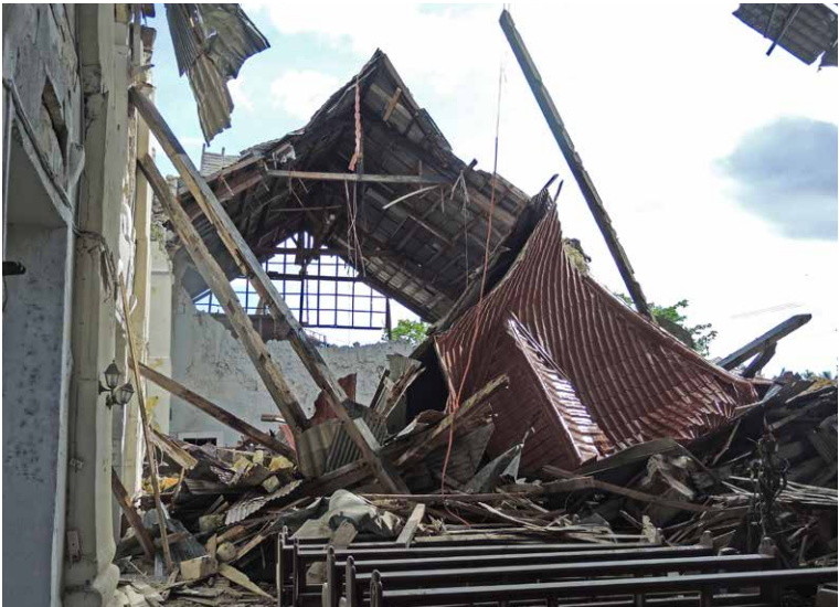
A church damaged by earthquake in Bohol, Philippines, 2013. Photo: Aparna Tandon, ICCROM.
